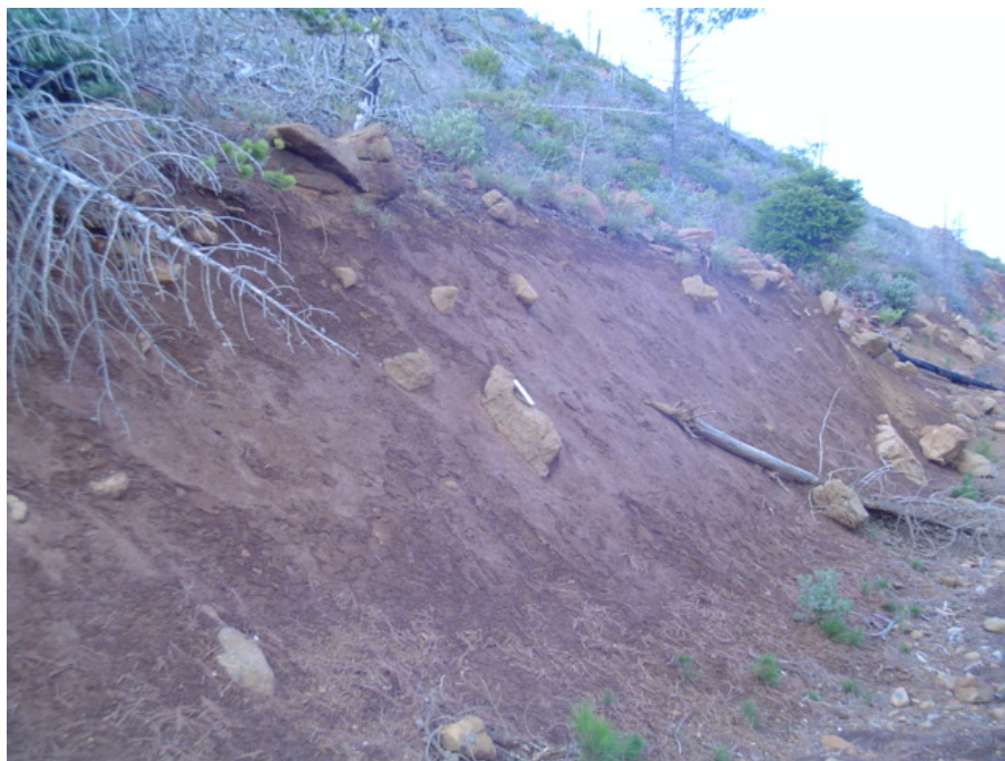
Figure 8. 4 - Road cut in possible sliding material near the southern part of the property
